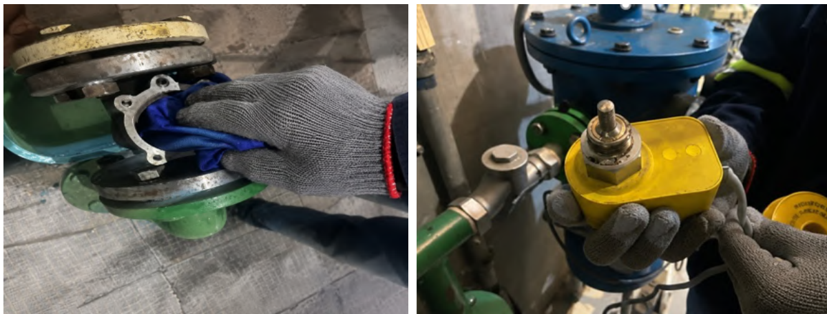
Figure 21 Cleaning of component during Unit #1 Quarterly Maintenance Activities
