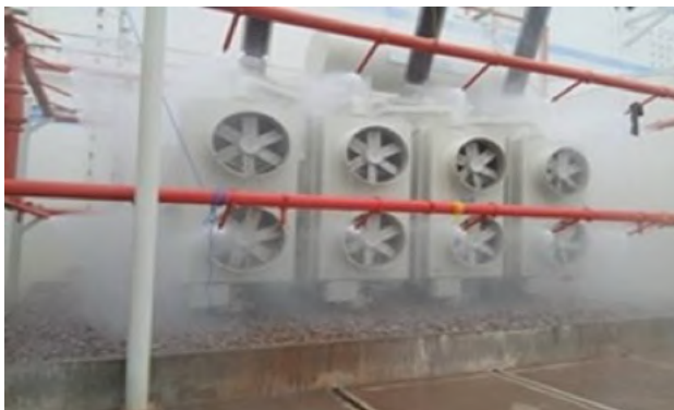
Figure 18 54G1- Functionality Test of the Deluge System
