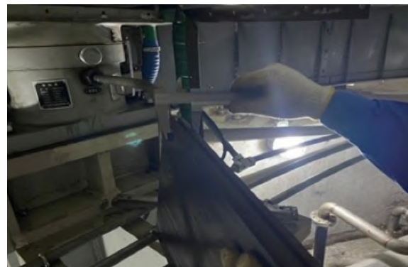
Figure 19 54G1- Measuring of the Brake Pad Thickness
